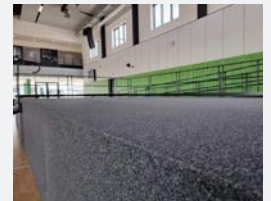
QUATTRO Fascia installed around Stage
